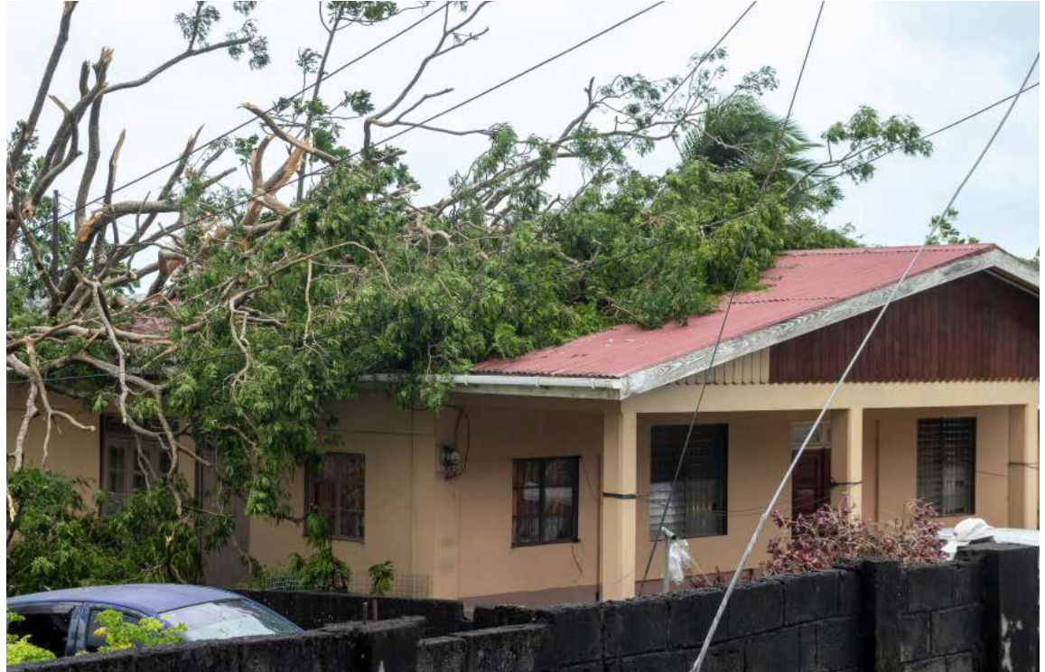
A tree lies on the roof of a house in Kingstown, St. Vincent and the Grenadines, after Hurricane Beryl on Monday, July 1, 2024. Photo: AP/Lucanus Ollivierre
