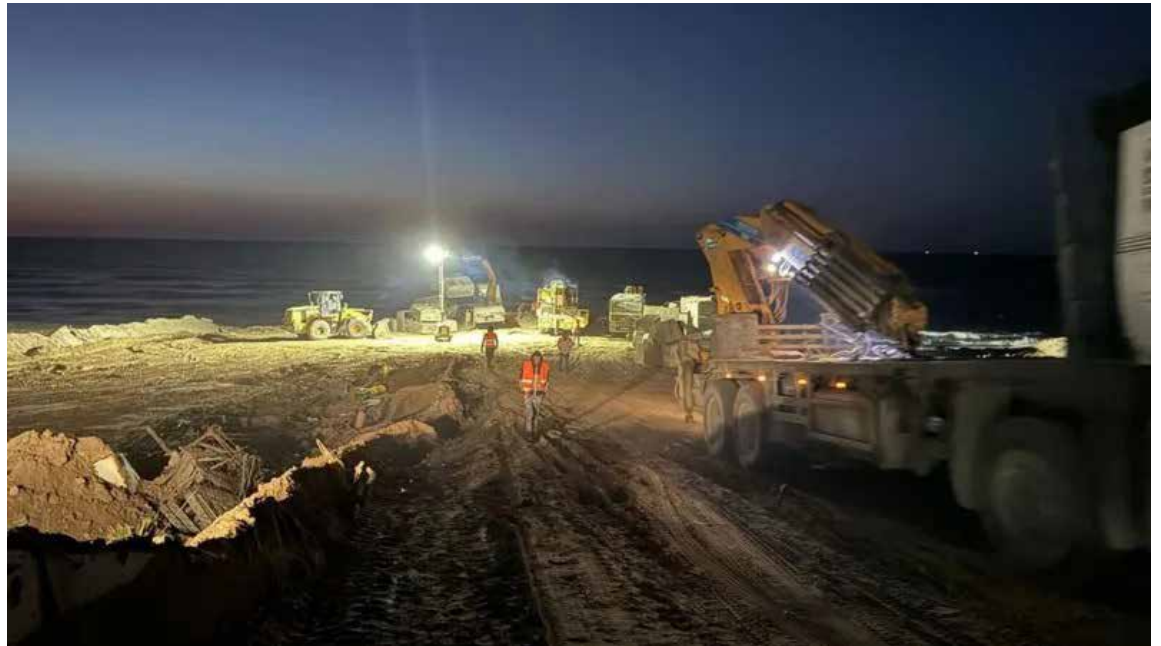
World Central Kitchen founder Jose Andres posted a photo showing workers building a jetty on Gaza's coast.
