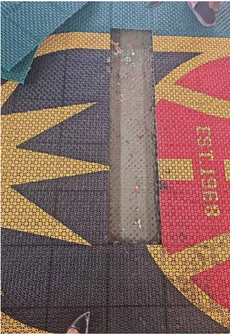
Repairs are being made to fix the part of the basketball court that was vandalized at the JSC Sports Complex.
