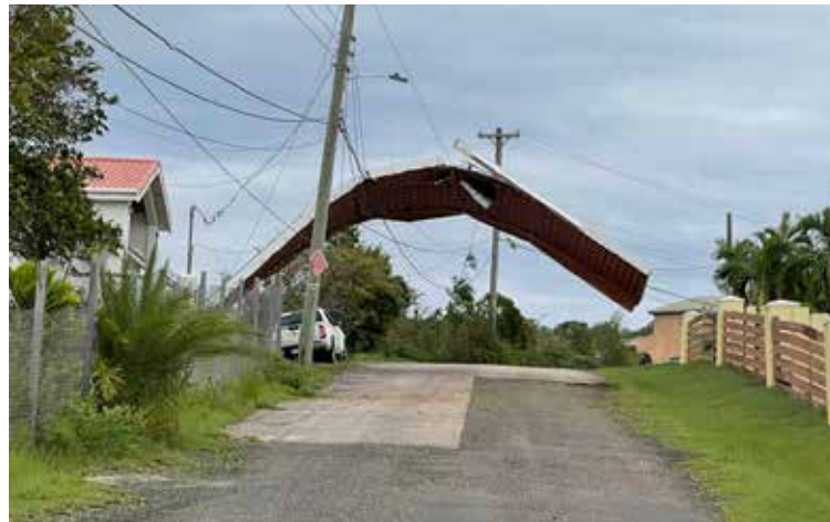
A galvanise sheeting from a house roof in Liberta landed on the electricity wire.
