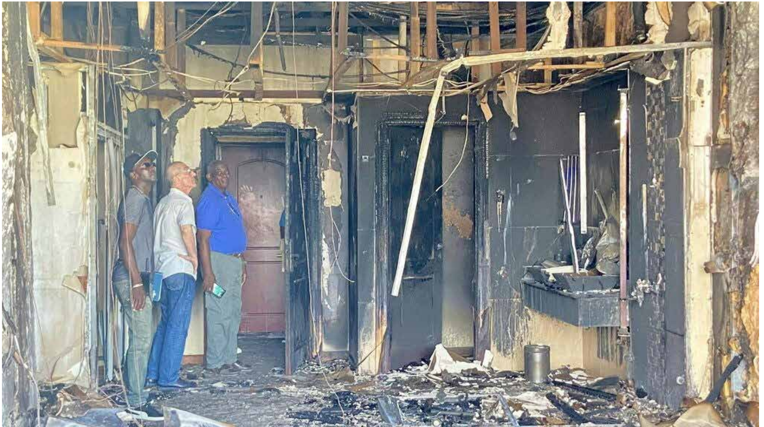
Officials examine the damage in one of the rooms at the Ramada Princess Hotel and Casino where a fire broke out on Saturday night. (Photo: Newsroom & Ministry of Home Affairs)
