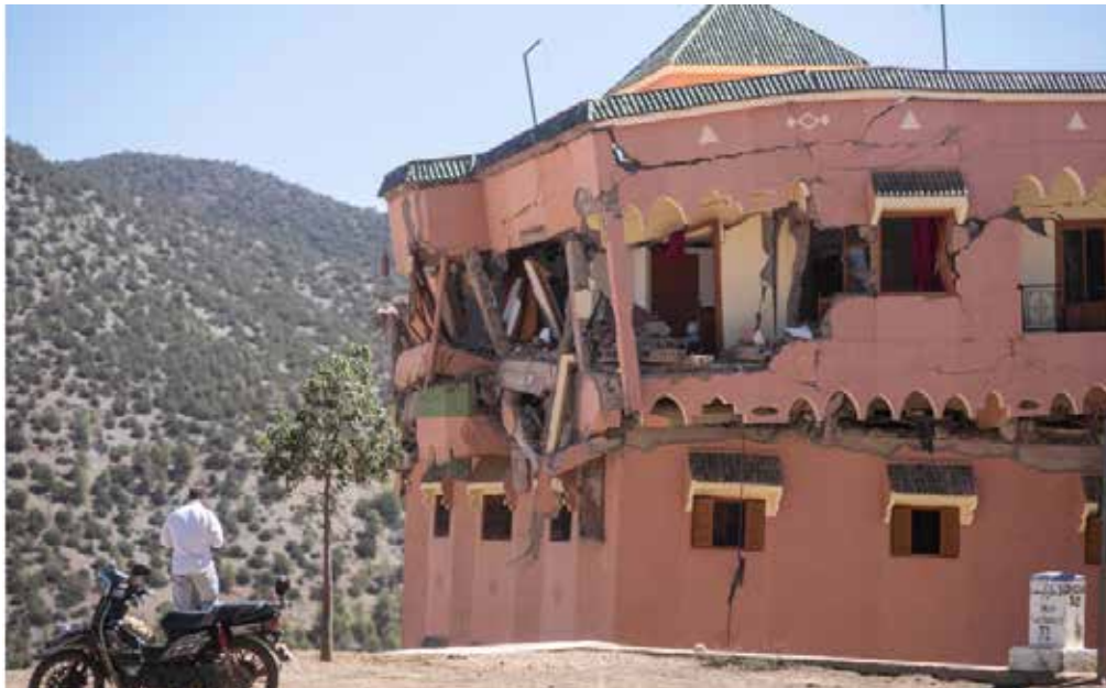
A man stands next to a damaged hotel after the earthquake in Moulay Brahim village, near the epicentre of the earthquake, outside Marrakech, Morocco, Saturday, September 9, 2023. (AP Photo/Mosa'ab Elshamy)
