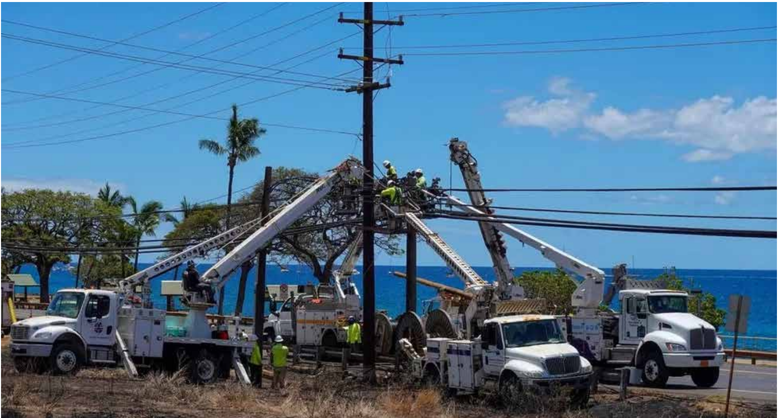
Witnesses say they saw sparks from power lines which ignited fires during a hurricane.
