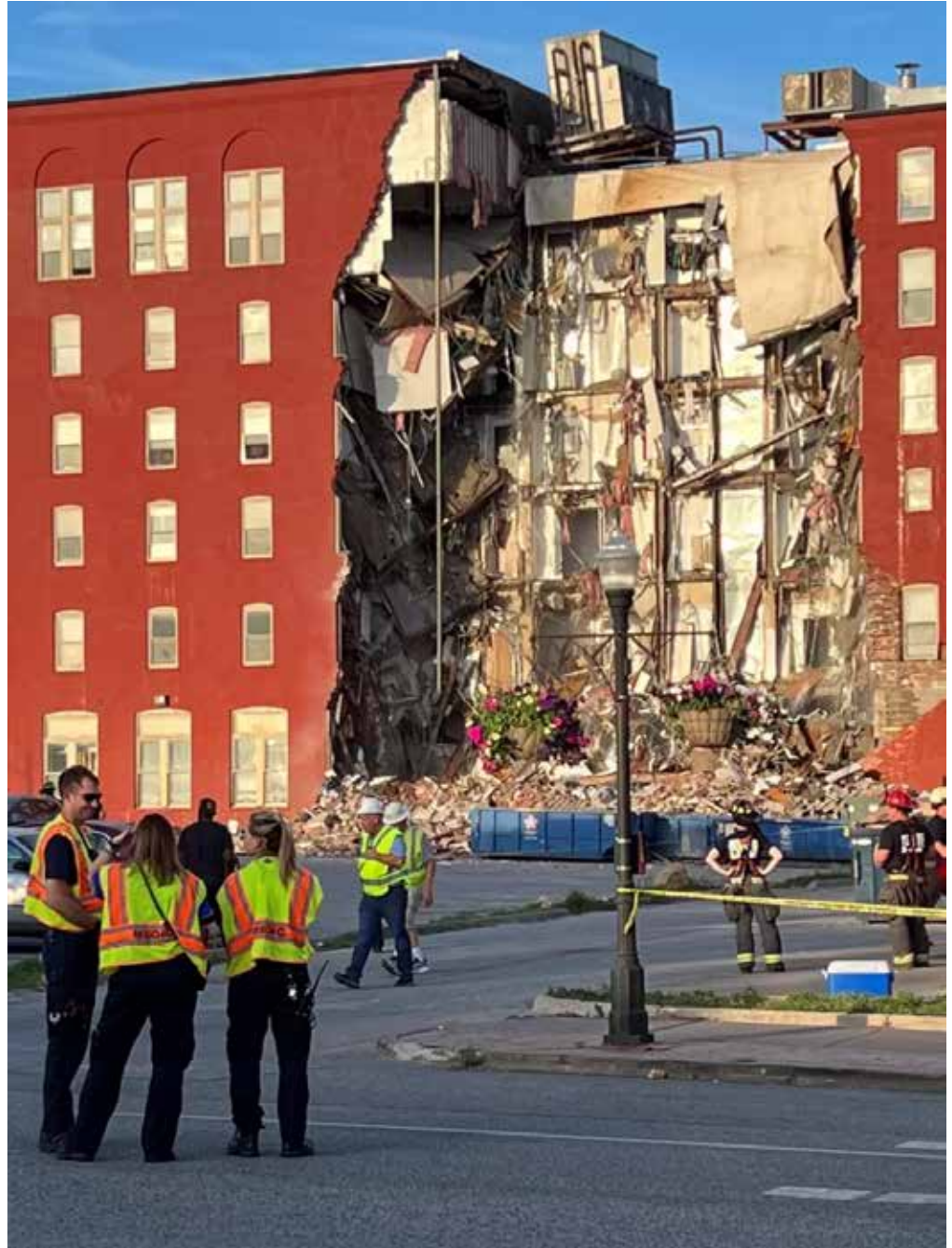
Local officials believe the building is at risk of collapsing entirely.
