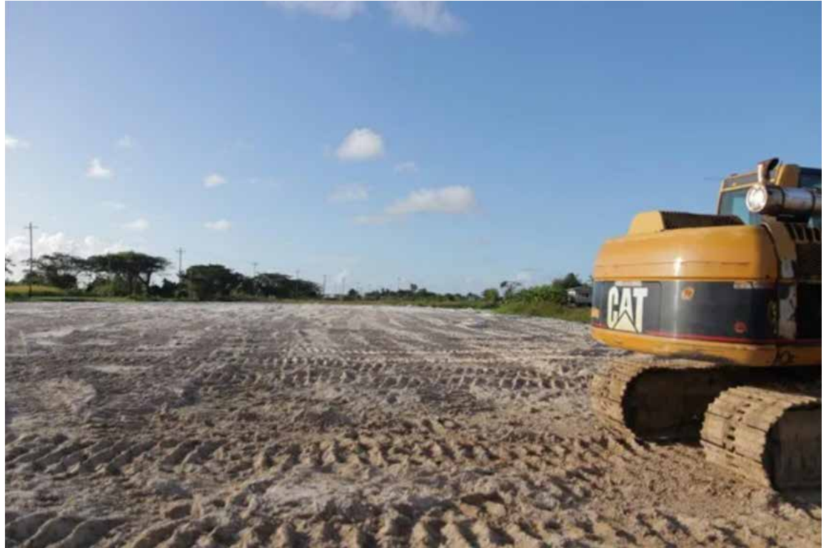
Heavy equipment stationed at one of the six new hospital sites. Photo via DPI.
