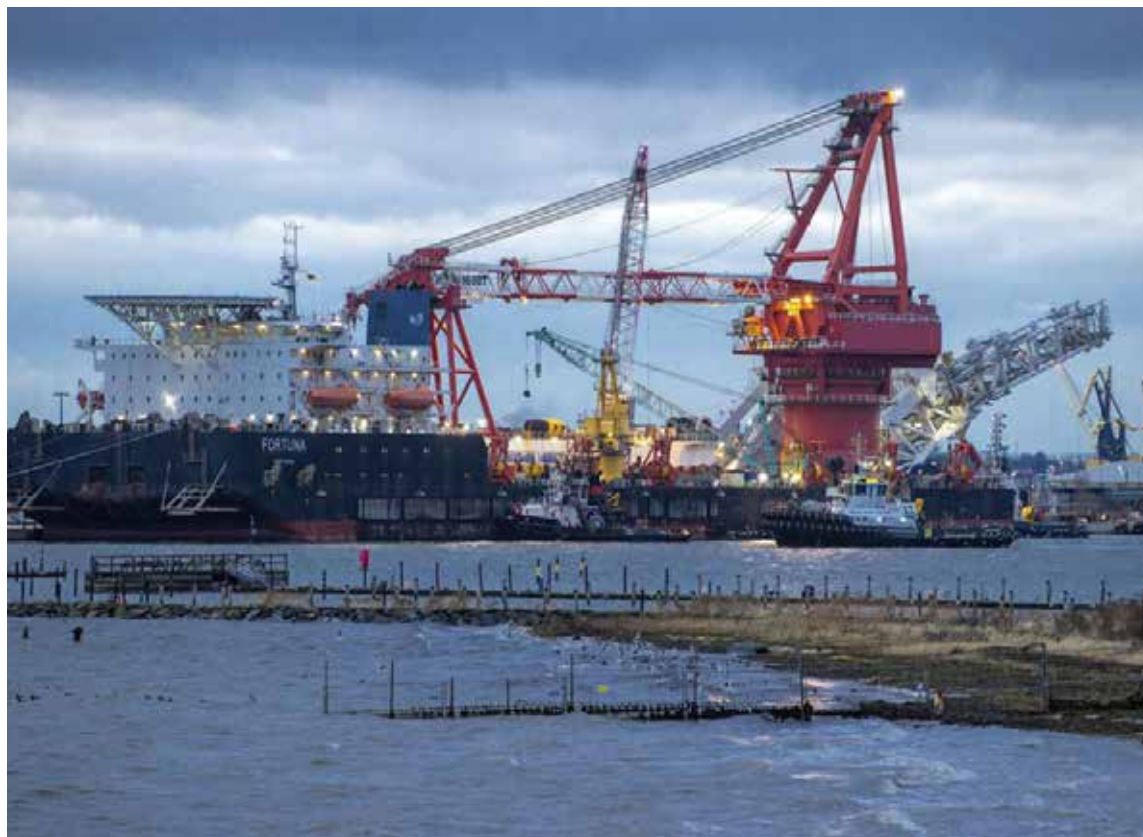
A tugboats get into position on the Russian pipe-laying vessel "Fortuna", being used for construction work on the German-Russian Nord Stream 2 gas pipeline in the Baltic Sea, in the port of Wismar, Germany, on Jan 14, 2021. European leaders are turning to Africa for more natural gas as the EU tries to replace Russian exports amid the war in Ukraine. (Jens Buettner/dpa via AP, File)
